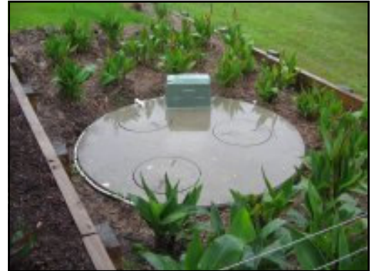
This home owner has landscaped around the Krystel Kleer treatment tank.
